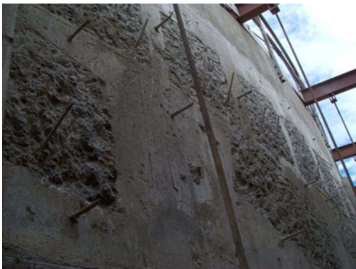
Figure 9. Face of the ring beam with box-outs after removal of a section of the concrete overlay.
