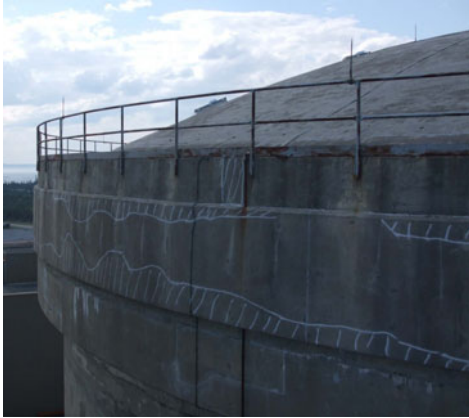
Figure 3. Delamination of non-structural concrete overlay of the ring beam.
