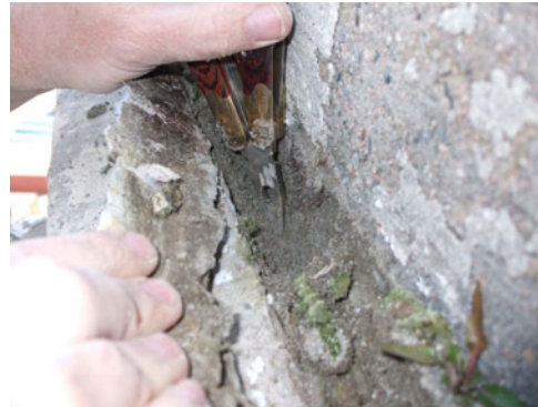
Figure 2. Configuration of joint top concrete overlay showing sealant failure.
