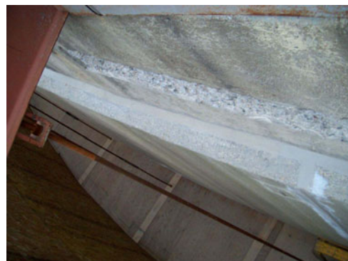
Figure 8. A shallow repair area above the joint between the concrete overlay and the ring beam and repair sealant.
