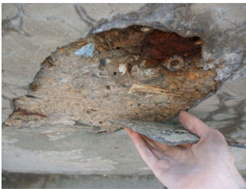
Figure 5. Embedded contamination on soffit of lower ring beam including foam insulation, wood chips, saw dust, steel nut and nails.
