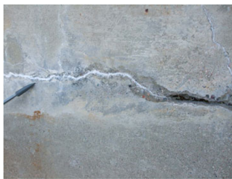
Figure 6. Crack filled with mineral deposits in the ring beam.
