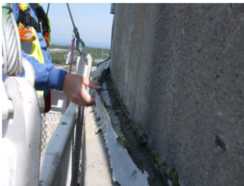
Figure 1. Failed sealant at joint between the top of concrete overlay and upper RB ring beam.
