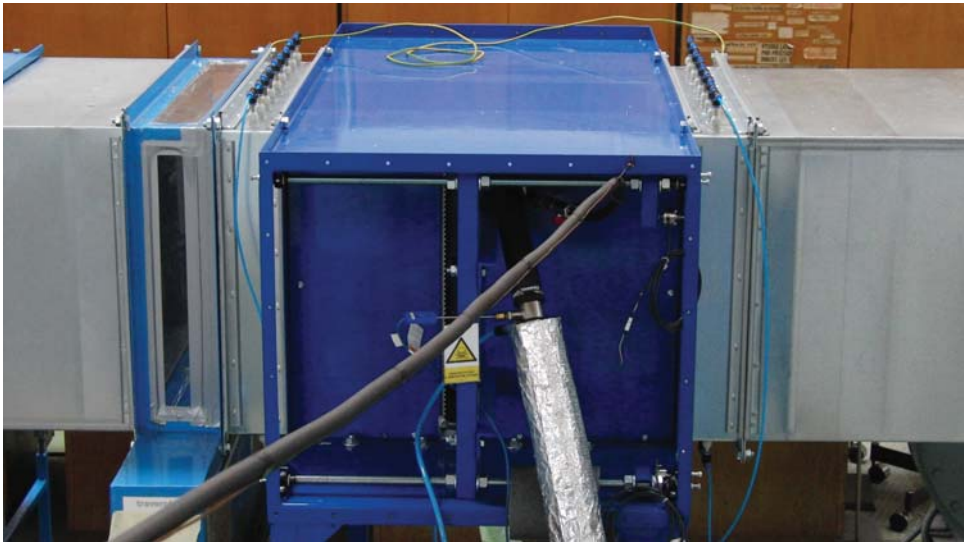
Figure 2: Measured heat exchanger in the measurement area
