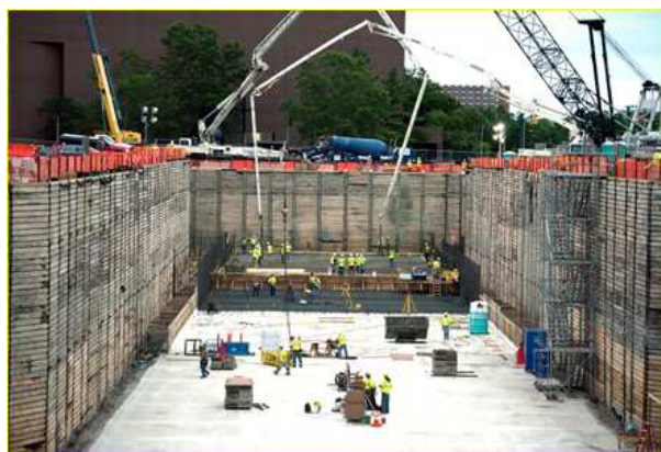
Figure 5. Photograph of FRIB's first foundational concrete being poured on July 23 rd , 2014. The eastward view toward the future position of the ion source shows the subsurface space that will house the linear accelerator. Real-time images of the FRIB construction site can be found at Ref. [18].
