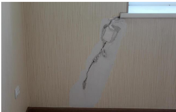
Fig. 6. Examples of cracks that formed in the stress concentration zone in the corner zones of window.
