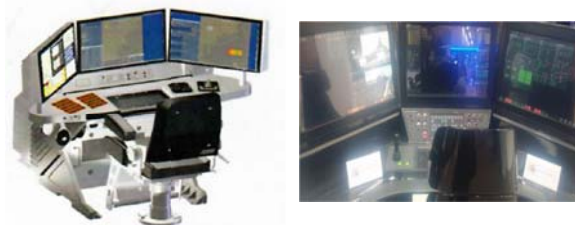
Fig. 2. Multifunctional control stations
