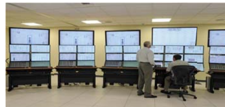
Fig. 1. Local control stations of the SMR
