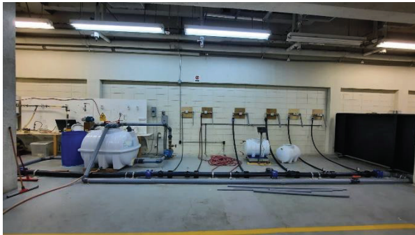
Fig. 1. System Set-up as installed in the Fluid Mechanics Laboratory – KFUPM.
