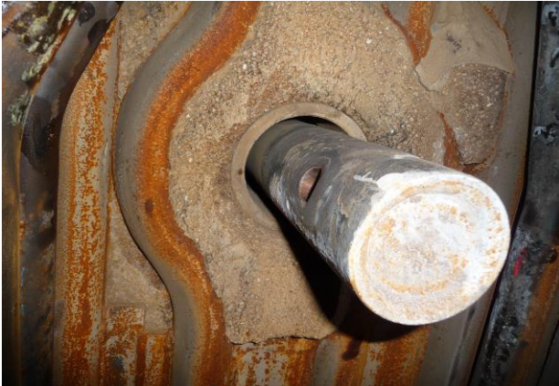
Fig. 2. Lance of retractable soot blower – inside boiler.
