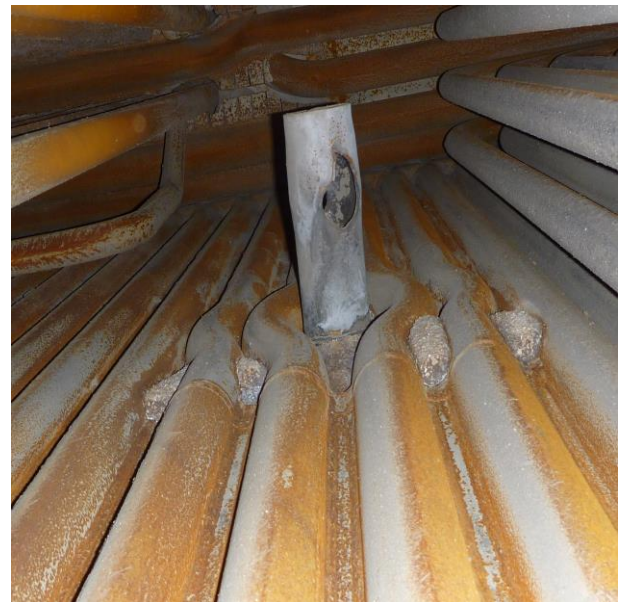
Fig 3 Overheat damage in a retract blower.
