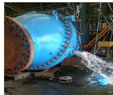
Fig. 4. Failure observed at high shaft bush leak.
