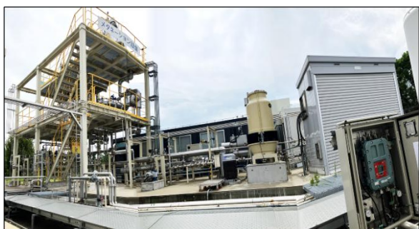
Fig. 14. OHC-800 deployed in a methanation plant.
