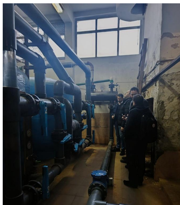
Fig. 2. Indoor thermal storage tanks (2 × 4000 l) and piping network of the GSHP installation at UTCN Swimming Complex, Cluj-Napoca.
