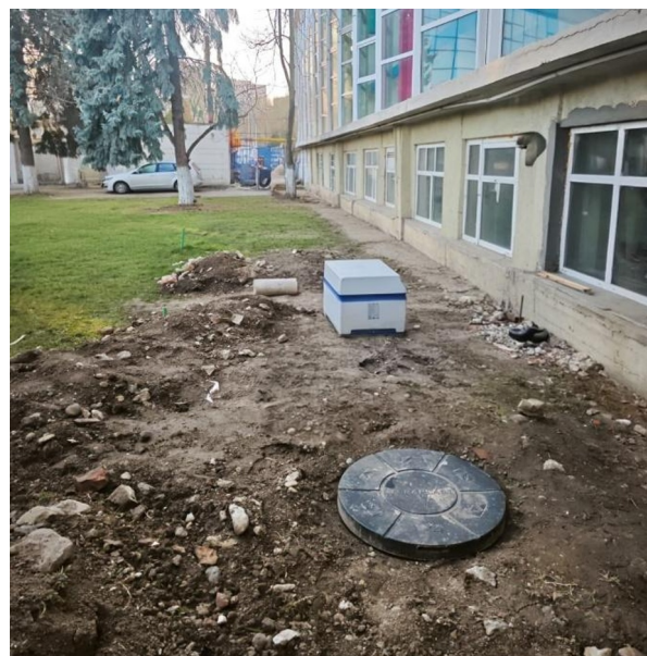
Fig. 1. Outdoor ground source heat pump unit (20 kW) and borehole access point connected to the 4 × 100 m vertical ground heat exchanger array at UTCN Swimming Complex
